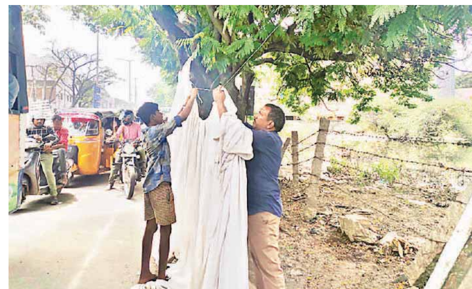
Workers hang up cloth sheets to cover up the sides of the route to Bapu Ghat
