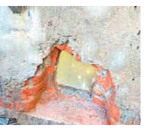
The hole made by the robbers to gain entry into the shop
