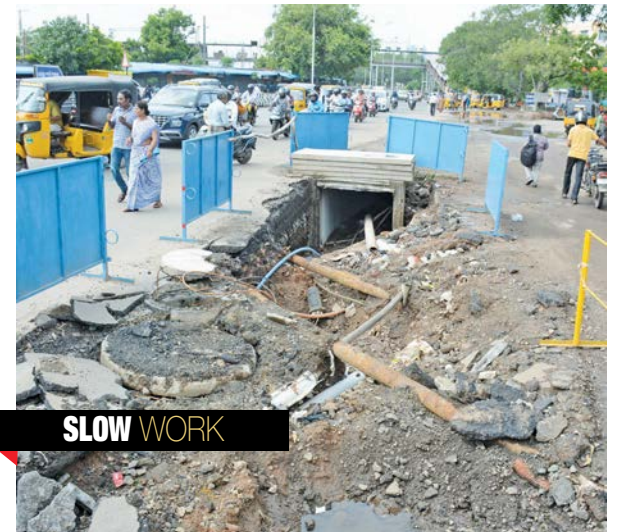
Stormwater drain work going on at slow pace in Parry's corner. —DC
