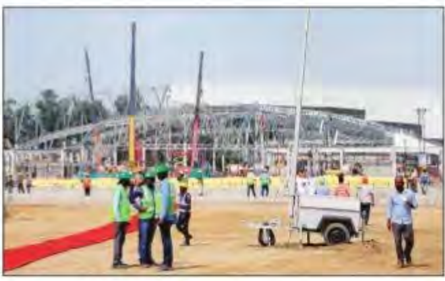
Construction work underway for the Kartarpur Corridor at Dera Baba Nanak in Gurdaspur, Punjab. PTI
