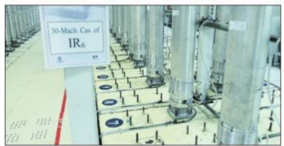
Centrifuge machines at Natanz uranium enrichment facility in central Iran. AP
