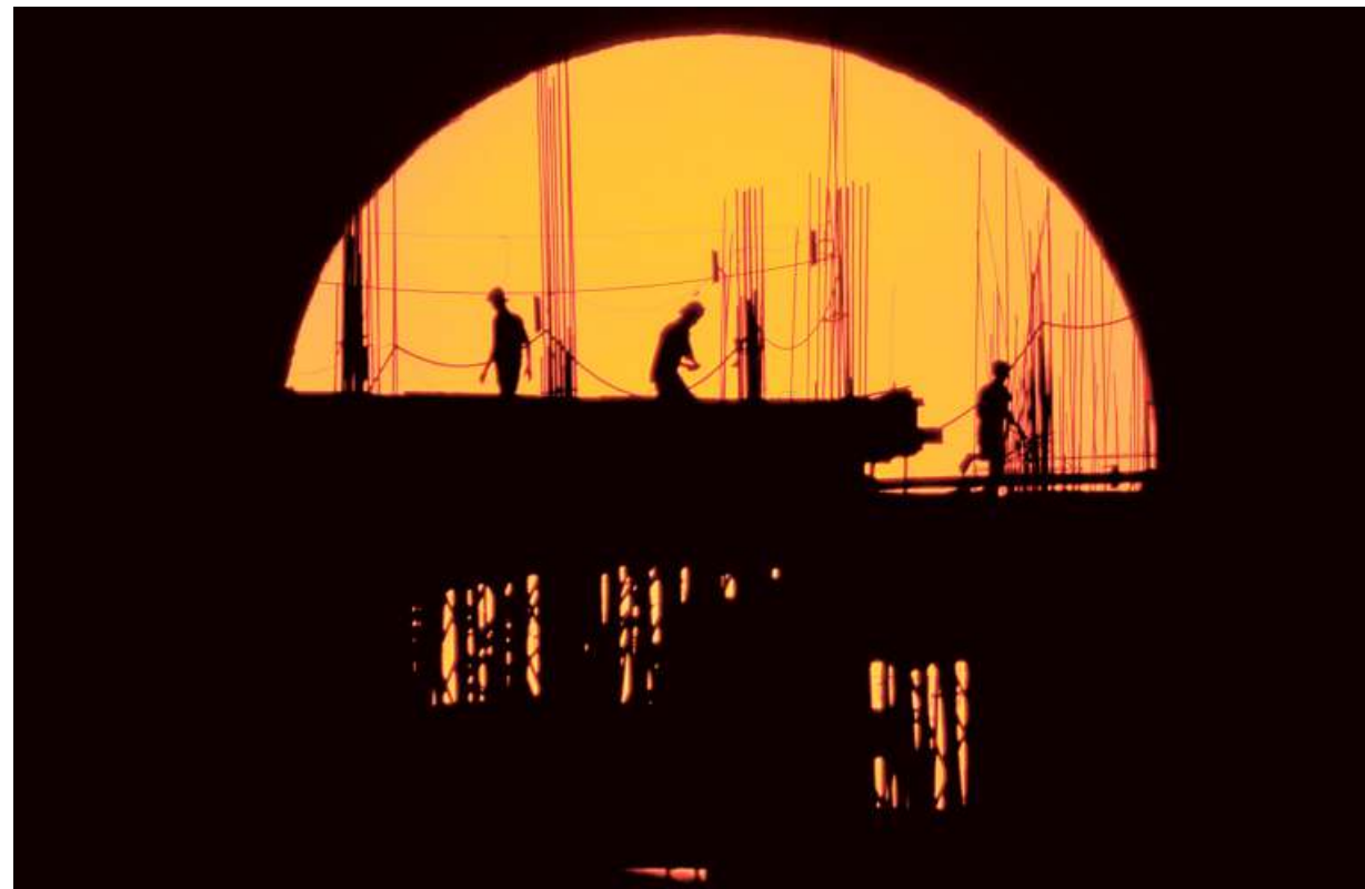
Workers engaged in construction work in Visakhapatnam on Wednesday. Building activity has picked up pace in Andhra Pradesh with the availability of sand improving after a prolonged shortage. ♦♦♦ K.R. DEEPAK
