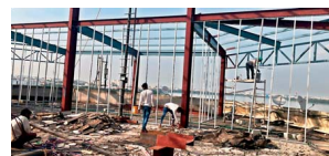
Works for a new office of the Chief Minister on the ninth floor of BRKR Bhavan underway.
