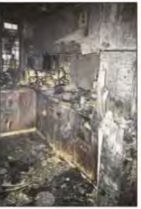
The fire started from the ground floor of the four-storey building
