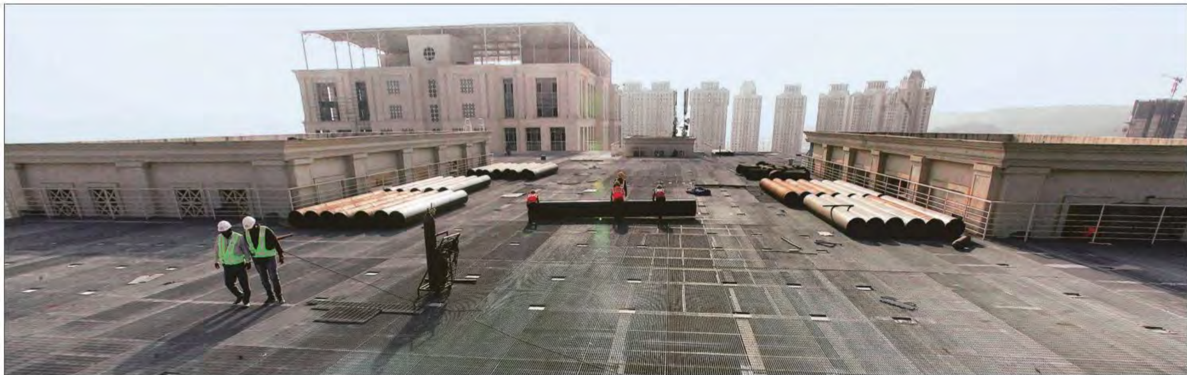
Construction on to build the country's largest ever data centre in Panvel, Navi Mumbai. The Rs 1,000-crore, 12-storey NM1 tower will hold 7,200 'data racks'. Pradip Das
