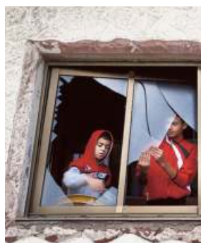
A home in Gaza City that was damaged following an Israeli attack on December 8. • AFP
