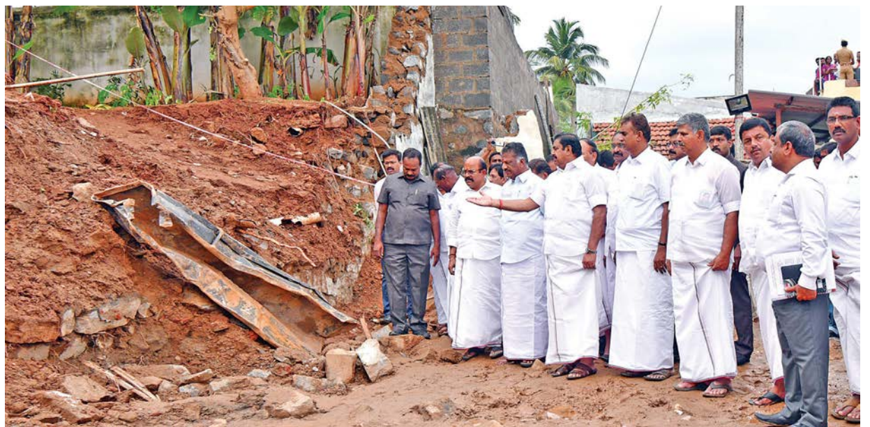
Chief Minister Edappadi K. Palaniswami and Dy CM O. Panneerselvam inspect wall collapse spot in Mettupalayam near Coimbatore on Tuesday.
