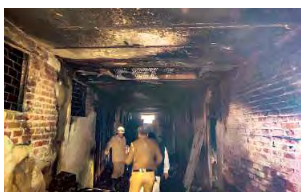
Police and rescue personnel inspect the gutted unit at Rani Jhansi Road in New Delhi on Sunday. ■ PTI
