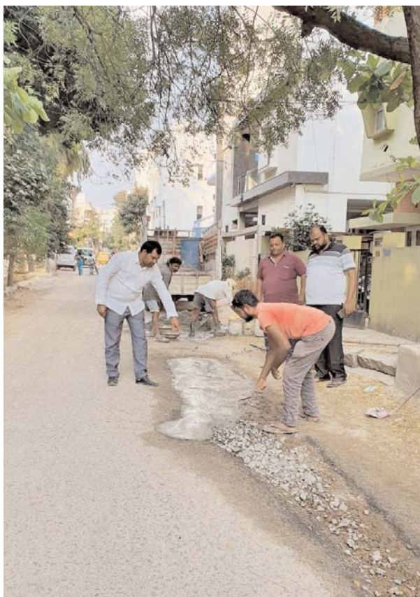
Residents repairing the road in the Secunderabad Cantonment as the board has said it has no money.
