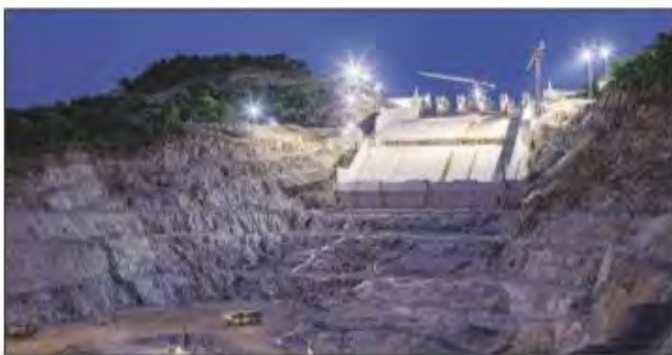
The Grand Ethiopian Renaissance Dam, under construction on the Blue Nile in Ethiopia. NYT
