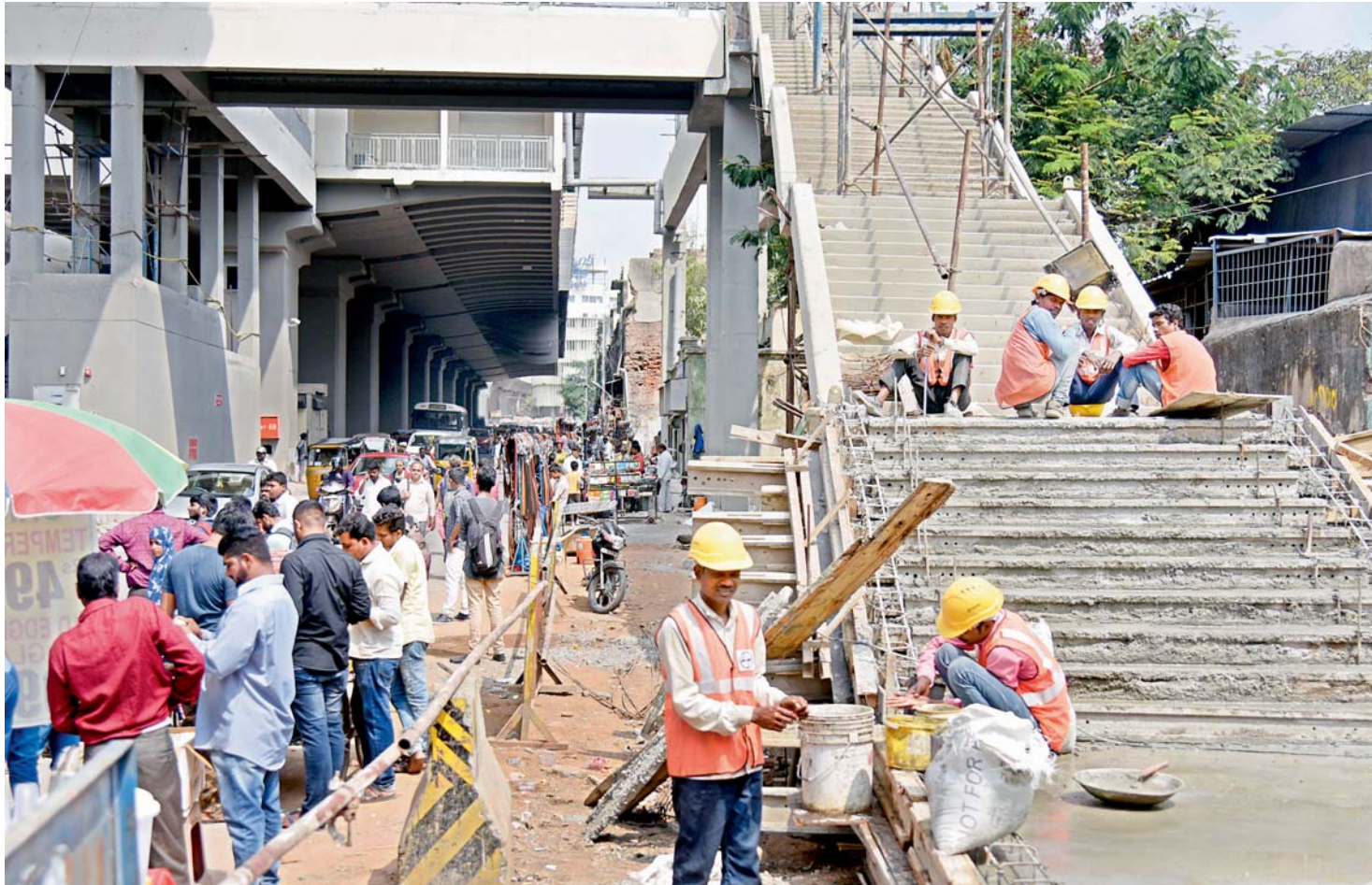
Works go on at the Sultan Bazaar Metro station which falls in the JBS-MGBS corridor which was inaugurated by Chief Minister K. Chandrababu Naidu last week. — S. SURENDER REDDY
