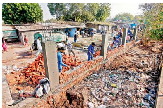
Workers construct a wall in front of a slum ahead of Donald Trump's visit to Ahmedabad.
