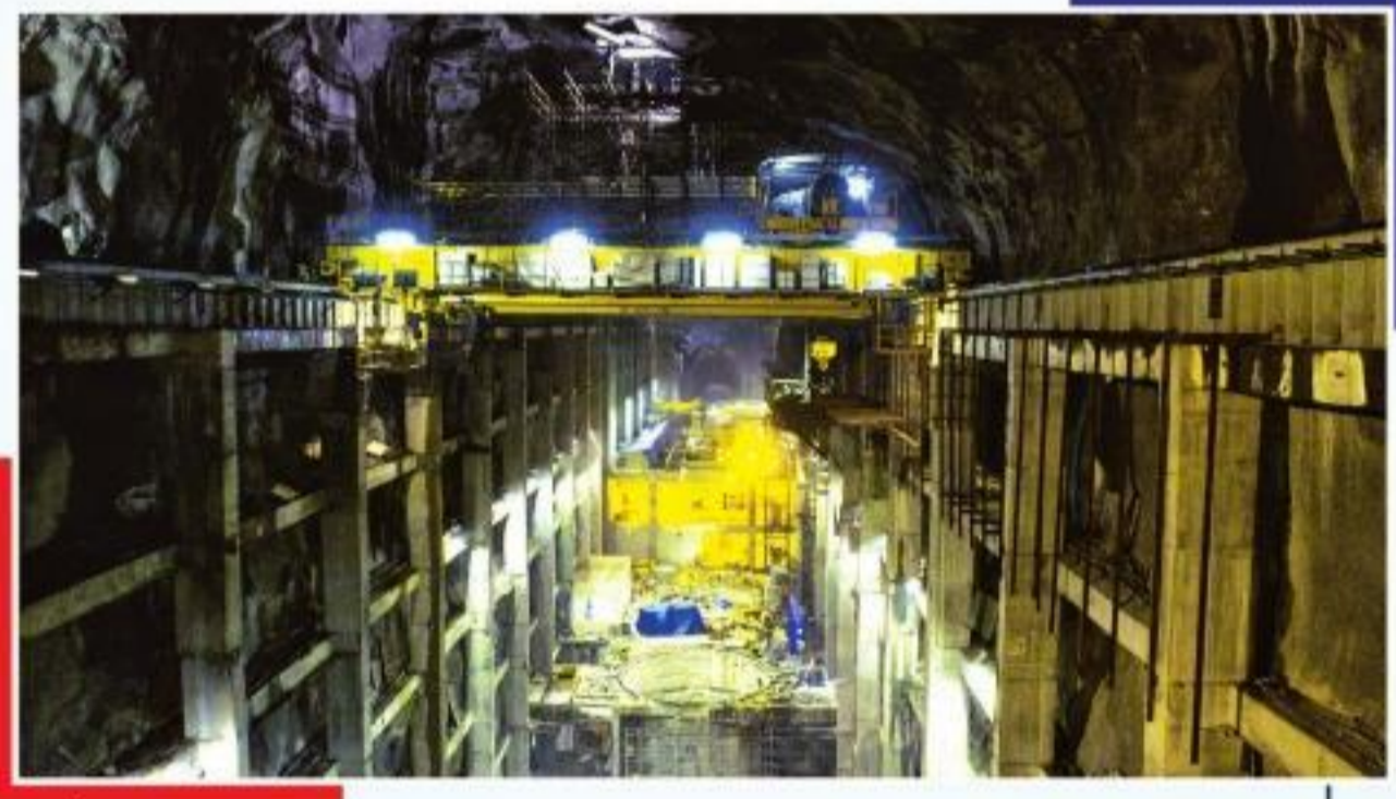
Kaleshwaram Pckg-8 Pump House
