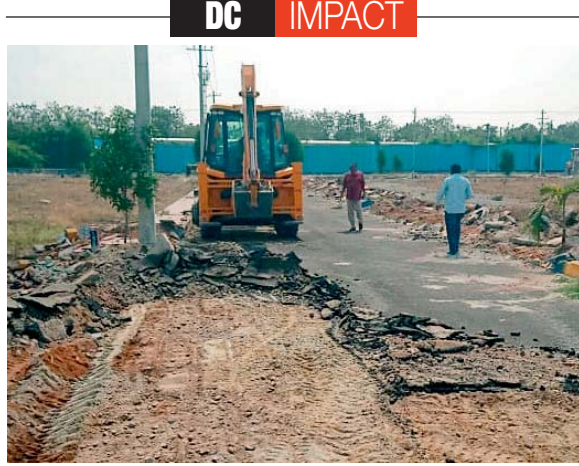
A JCB machine being used to demolish illegal layout constructed in full tank levels of Hussainsagar lake on Saturday.
