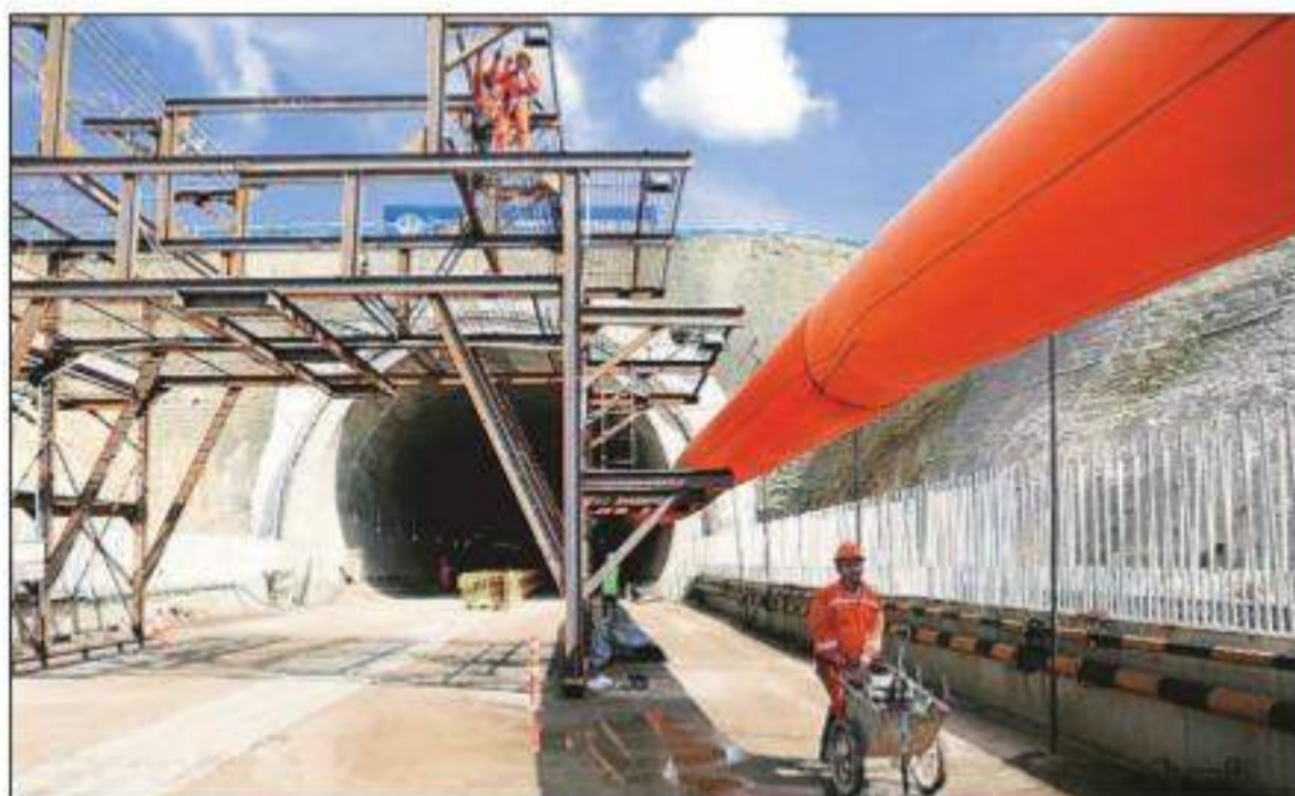
At Walini tunnel construction site for Jakarta-Bandung High Speed Railway in West Bandung regency of West Java province. The railway is China's flagship project in Indonesia. Reuters
