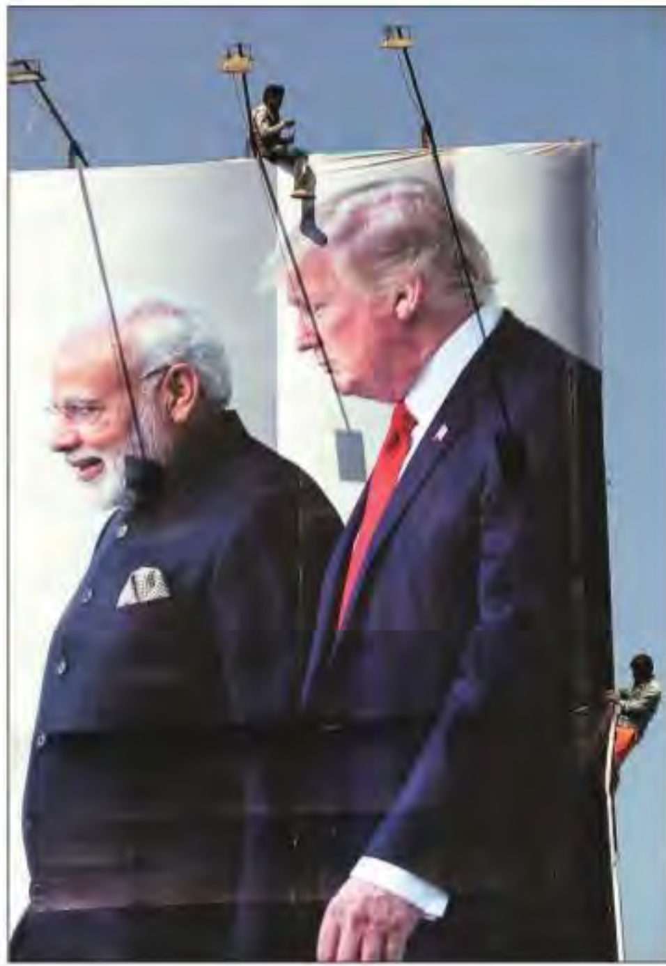
In Ahmedabad Thursday, workers put up a hoarding welcoming US President Donald Trump. AP
