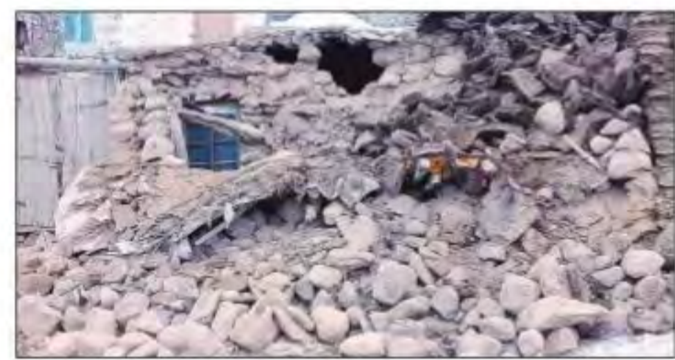
Houses are reduced to rubble after an earthquake hit villages in Baskale in Van province, Turkey. AP
