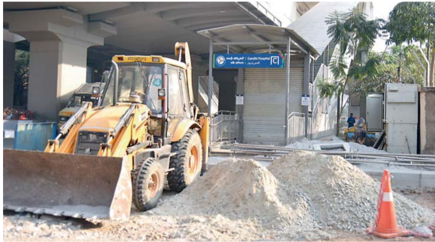
Works under progress at the Metro Rail station near Gandhi Hospital. — S. SURENDER REDDY.
