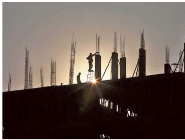
Dark days: Materials supply has stopped and sub-contractors are unable to arrange resources for construction activities
