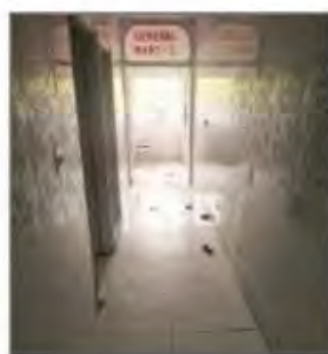
Windows were shattered on each floor. Gajendra Yadav
