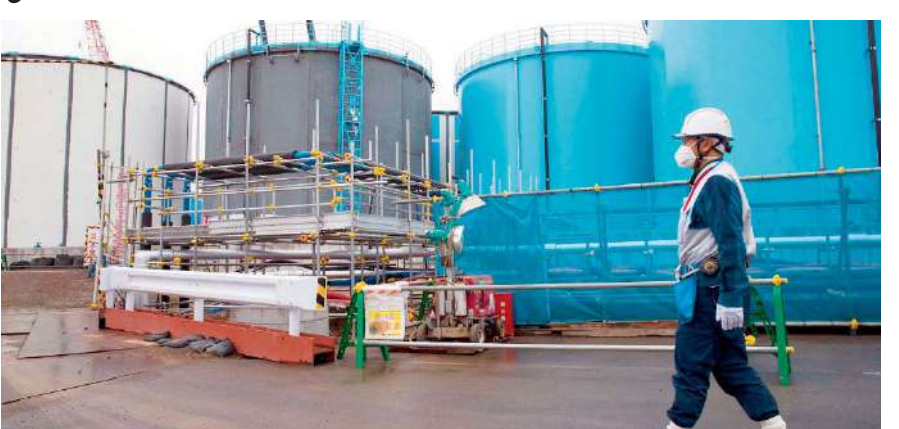
An employee walks past storage tanks for contaminated water at the Fukushima Daiichi nuclear power plant, Japan. — AP
