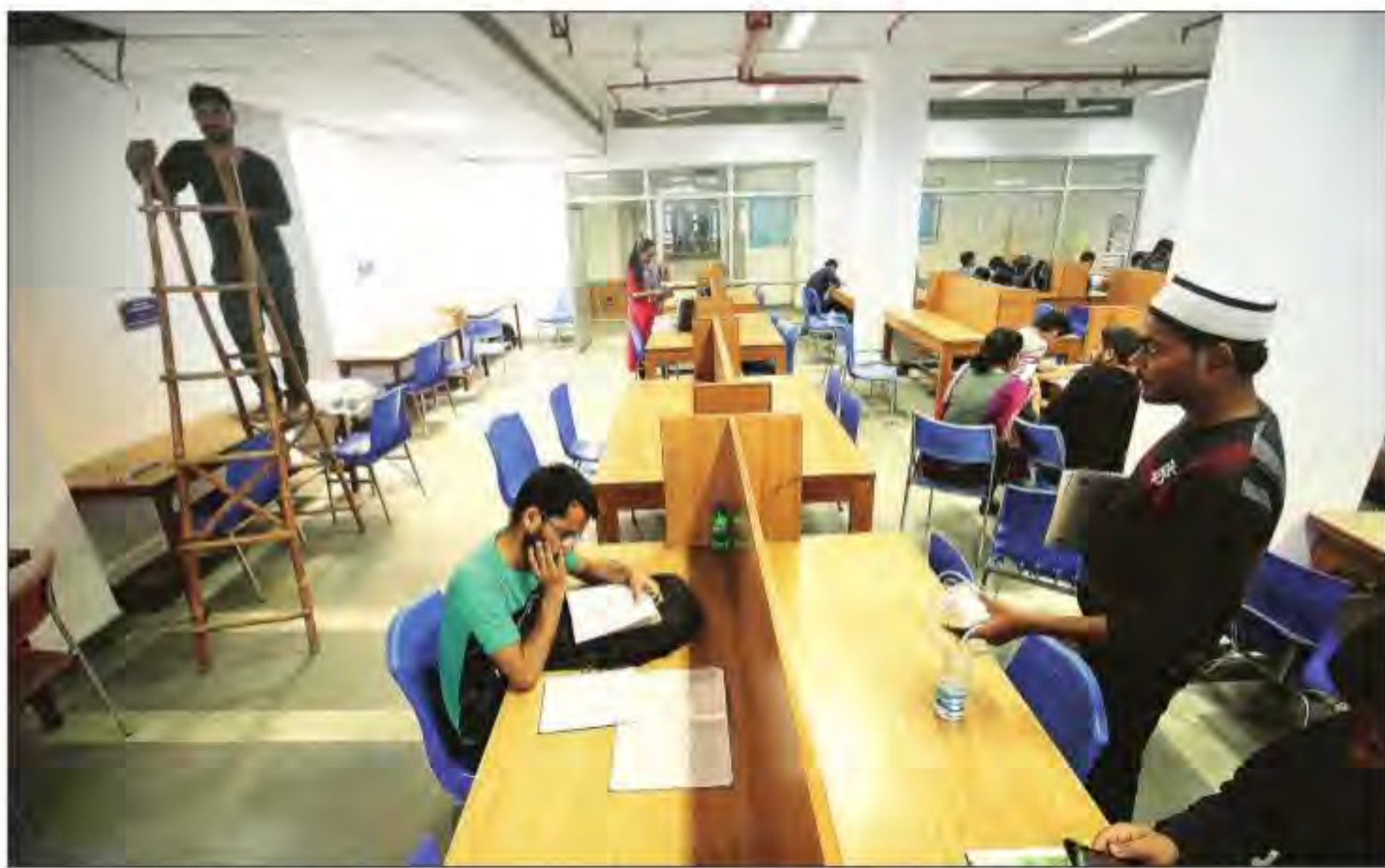
Renovation work continues as the reading hall in the New Library at Jamia Millia Islamia was opened Wednesday. The Old Library, which suffered the maximum damage, is yet to reopen. Praveen Khanna
