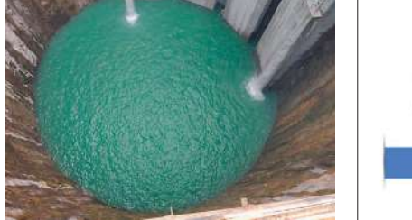
Asia's biggest Surge-pool constructed at Thimmapur village of Yellanthakunta mandal under KLIS project package 10. - DC
