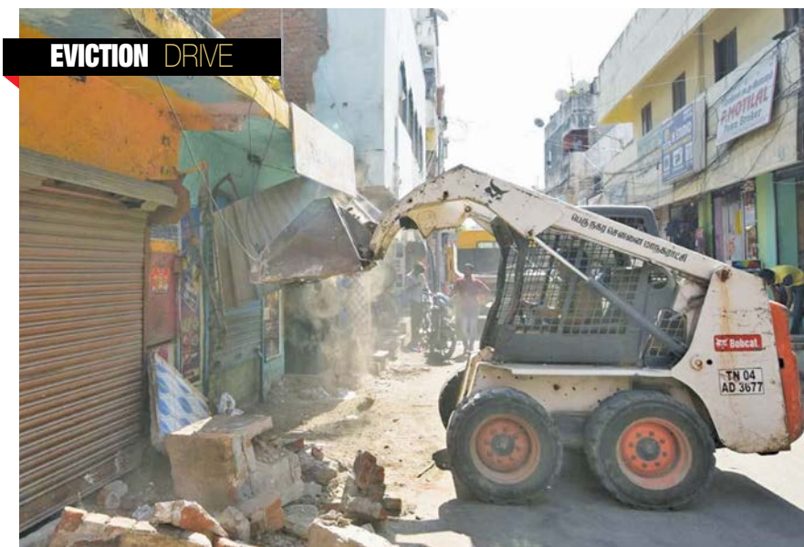
Greater Chennai Corporation staff demolishing an encroachment in Ashok Nagar on Thursday. —DC
