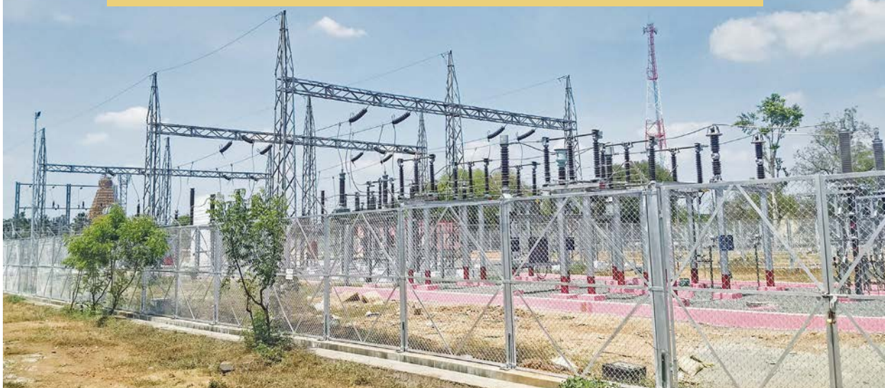
Electric sub-station at Thanjavur for railways.
