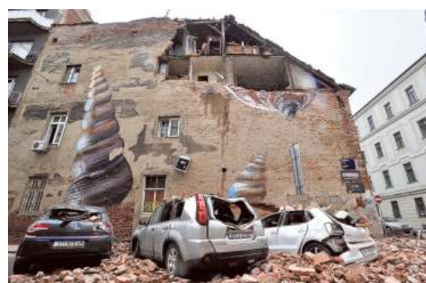
Double shock: A wall that collapsed due to the impact of Sunday’s quake in Zagreb, Croatia. •AP
