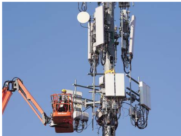
Companies have activated a comprehensive pandemic response plan with requisite risk mitigation protocols for keeping networks working as telecom is an essential service
