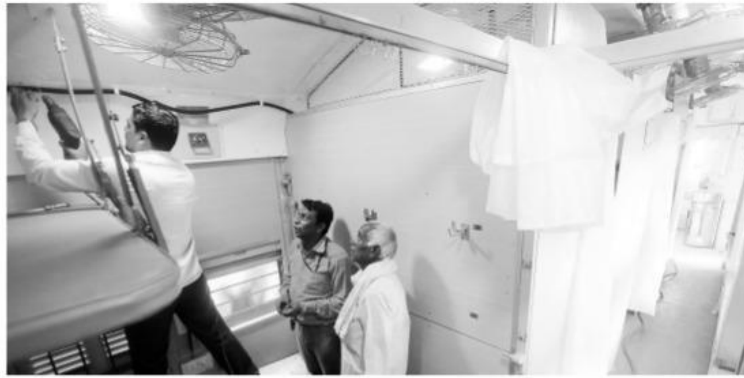
Workers alter the interiors of the train coach at New Delhi station. Tashi Tobgyal
