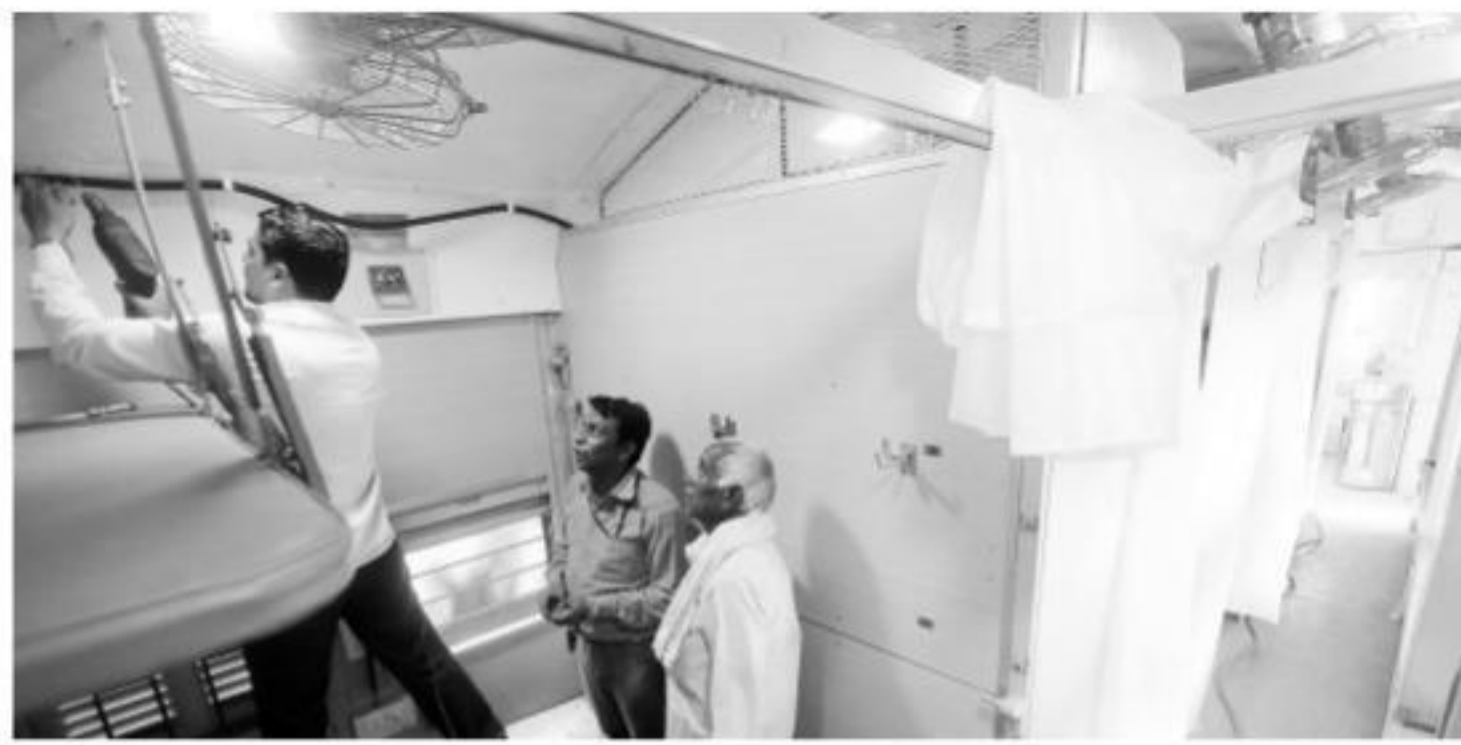
Workers alter the interiors of the train coach at New Delhi station. Tashi Tobgyal
