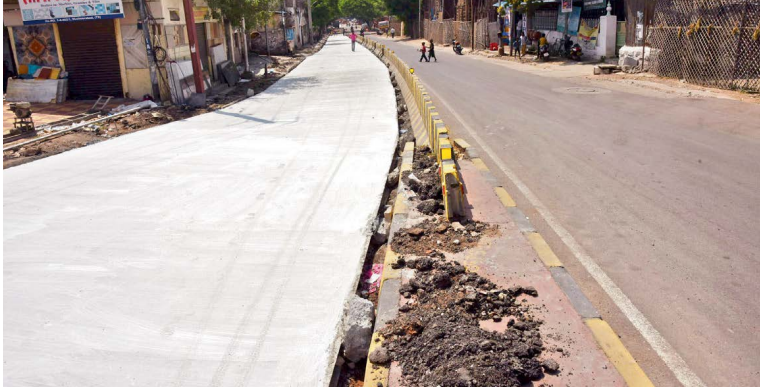
The lockdown due to Covid-19 pandemic comes in handy for the GHMC authorities to implement their decades-long-pending plan of laying a concrete road in the Kavadijuda corridor, one of the busiest routes, in Secunderabad, on Thursday. — GANDHI
